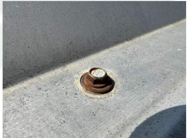
Close-up of fastener with deteriorated washer
