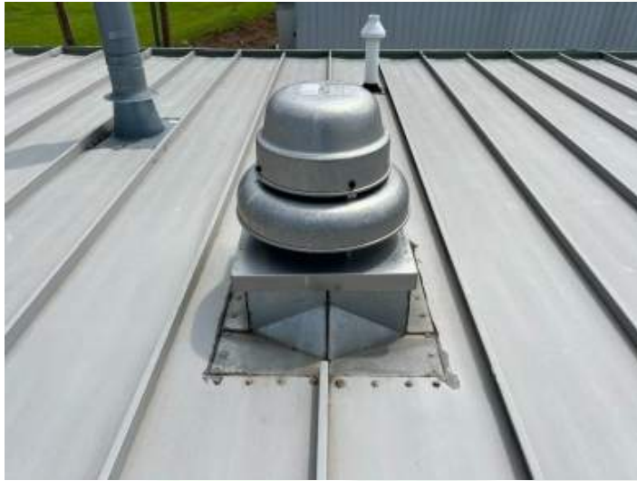
Roof penetrations are needing to be resealed
