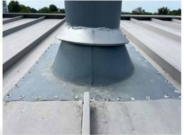
Penetrations span ribs in panels need to be sealed
