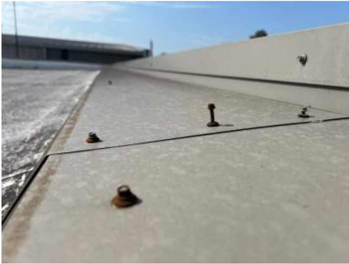
Backing fasteners shown at the seam of this panel
