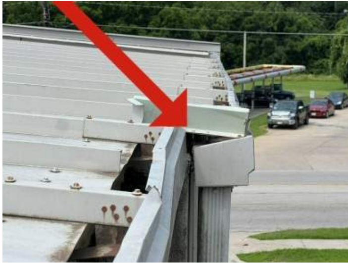
Detached gutter from previous photo roof surface view
