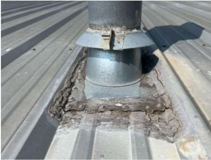
(2) pipe flashing bases not sealed
