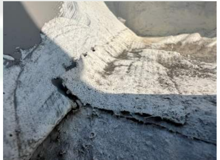
Tie in to metal is peeling and is need of repairs
