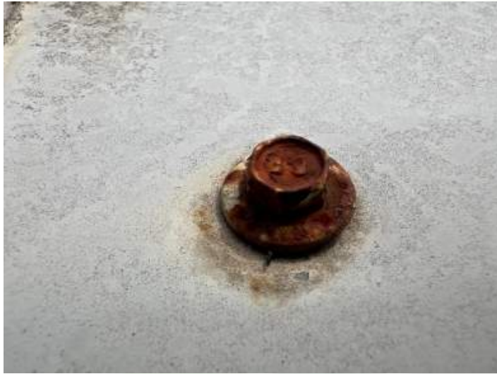
Rusting areas at failing fasteners
