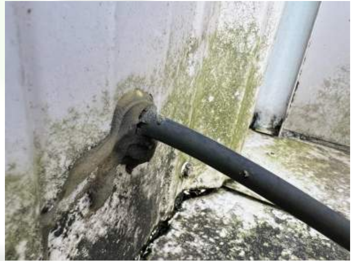
West wall line penetrating and not sealed
