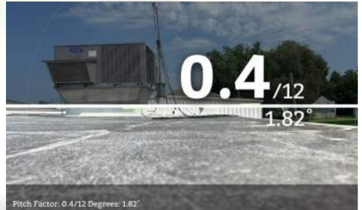
Less that .5"/12" structural taper to drain to lower roof section
