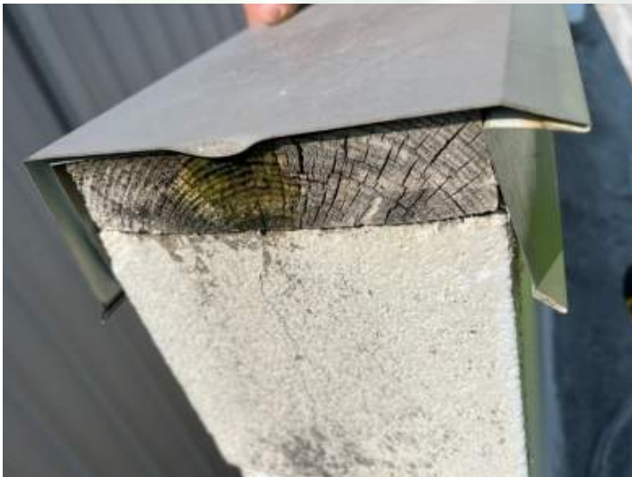
Missing End cap for coping on South wall
