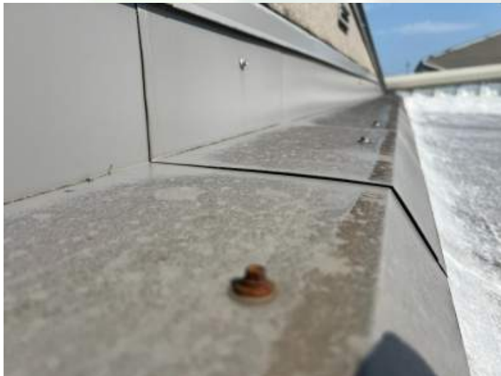
Top fasteners are backing up and failing on all flashings
