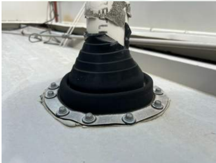
Pipe flashing damaged
