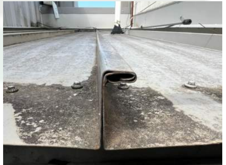
Mechanically crimped standing seam panel roof system
