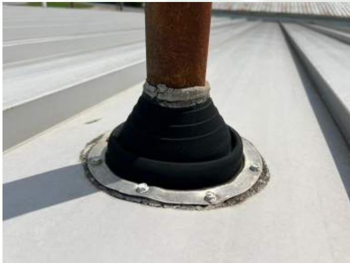
Pipe flashing improperly installed with more fasteners
