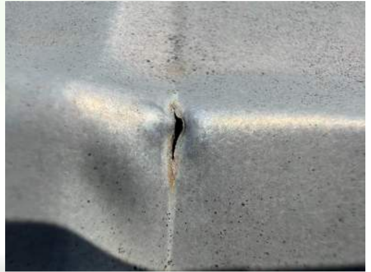
Fractures are found in the ridge cap from expansion and contraction
