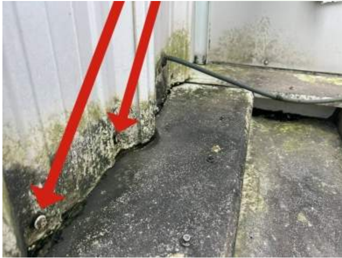
Loose fasteners observed at South wall
