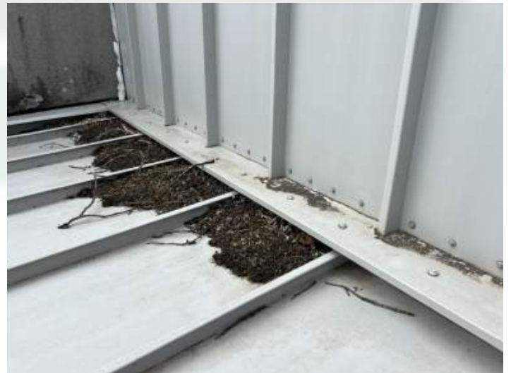
Debris in SW corner of the roof
