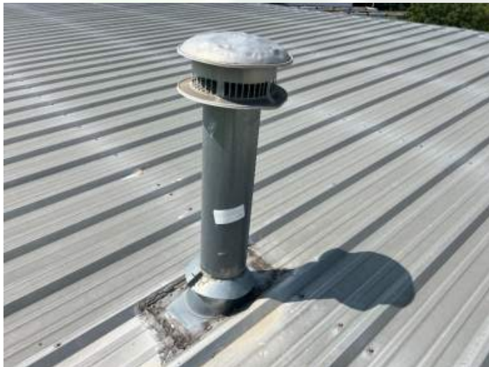
(2) pipe flues / Hail damaged caps
