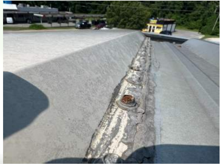
Fastener washers are deteriorated
