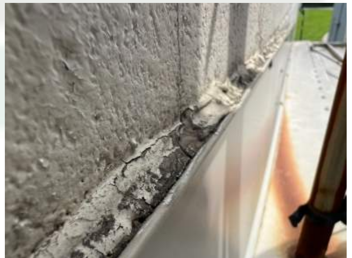
Sealant deterioration at wall tie in
