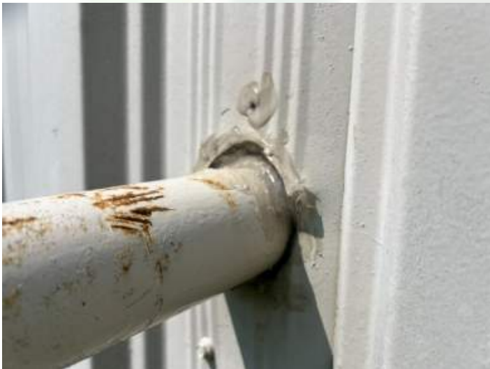
Wall penetration on East wall Close-up
