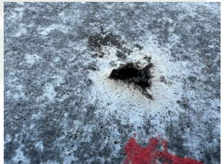
(1) area found in the roof field with damage to the coating
