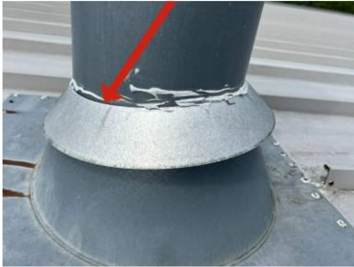
Storm collar is open to the driving rains
