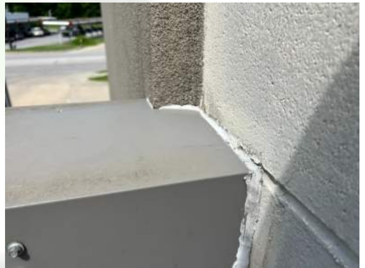
Coping cap seal deterioration
