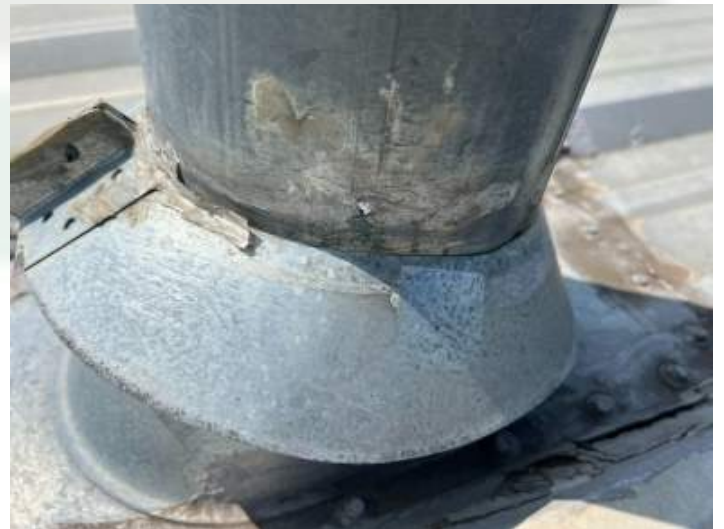
(2) pipe flue storm collars not sealed
