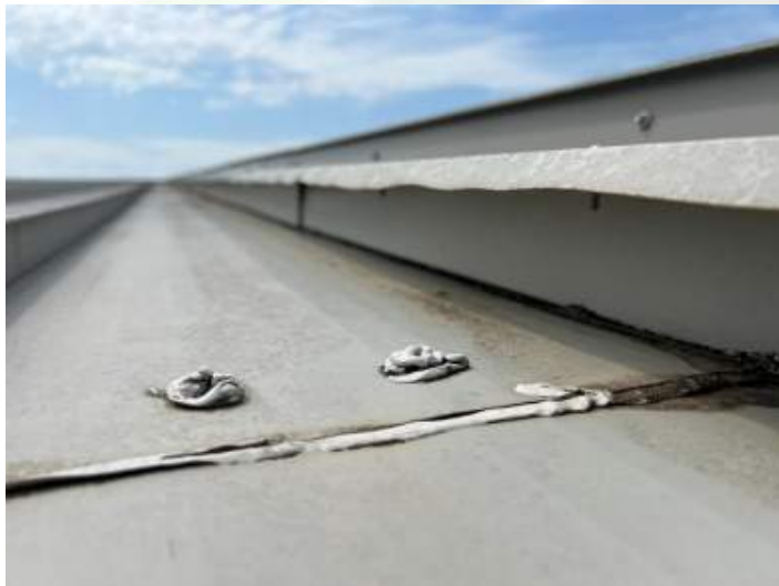
Previous caulked fasteners were found throughout
