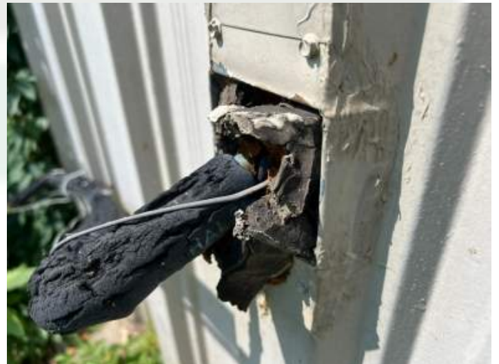
Wall penetration on East wall Close-up
