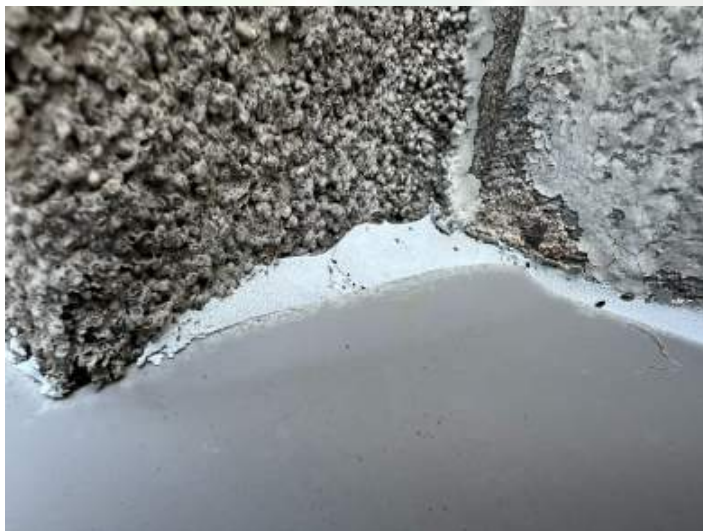
Close-up of sealant deterioration wall tie in
