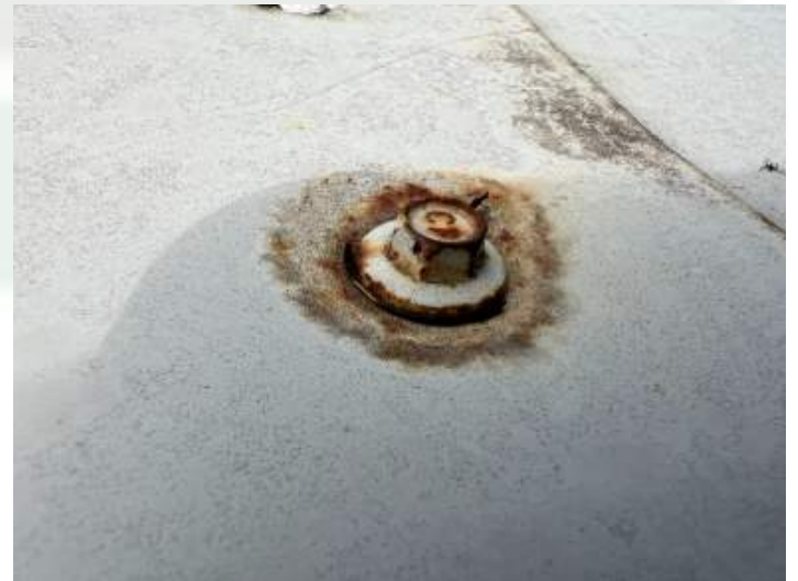
Rusting areas at failing fasteners
