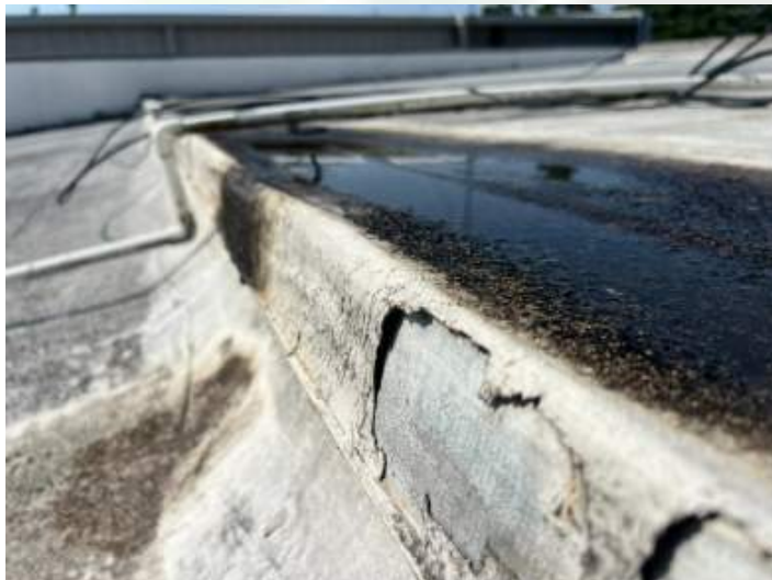
Peeling coating at upper section roof edge
