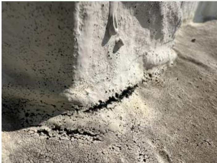
Close-up photo of defects on the North Perimeter
