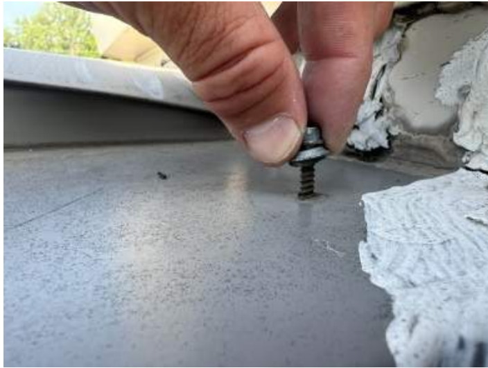
Fasteners are backing up on the top side of the metal flashings
