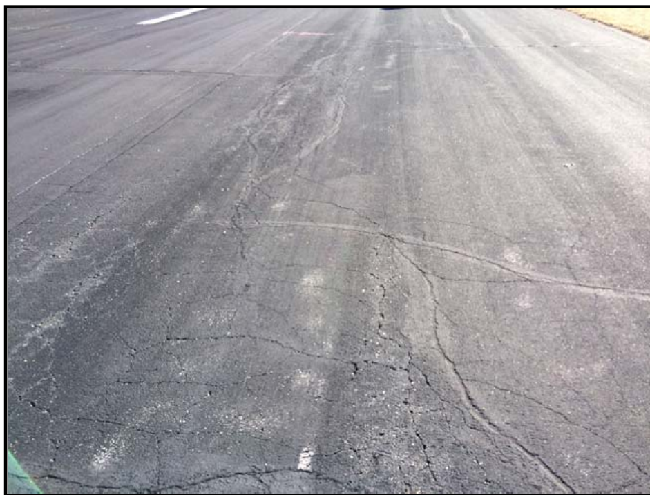
Photo 1: Runway 17-35 Pavement Cracking
