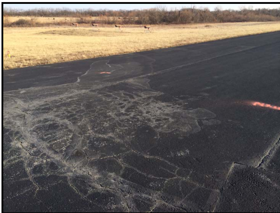
Photo 2: Runway 17-35 Pavement Cracking
