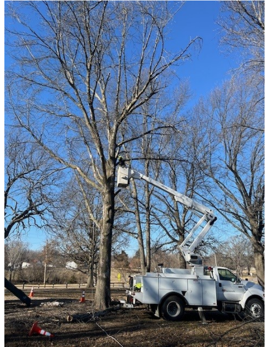
Tree removed at Shelter #2 in City Park
