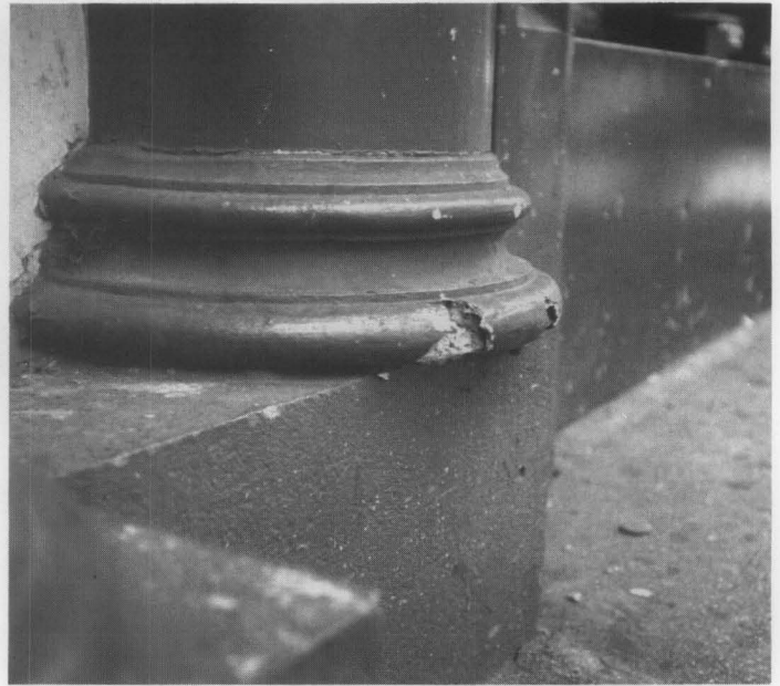
Fig. 20. The location of the feature must be taken into account if a substitute replacement material is being considered. This lightweight fiberglass column at street level sustained damage from impact within a few years of installation. The great strength of cast iron makes it ideal for storefronts and elements that must withstand heavy use. Photo: Building Conservation Associates.
