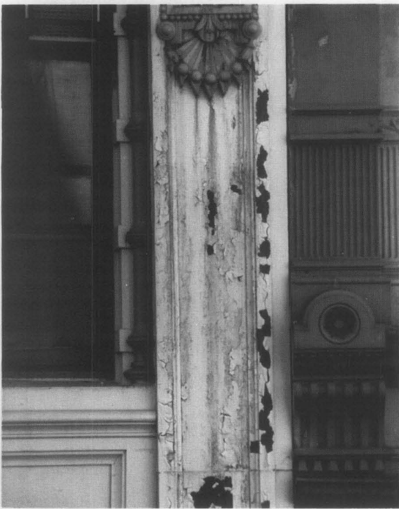
Fig. 14. Major problems can result if work is undertaken without proper sequencing and precautions. On this building, a strong alkaline paint remover was used, and apparently was not adequately rinsed or neutralized. Over a period of months, the newly applied paint began to peel and streaks of rust appeared on the iron. Photo: Kim Lovejoy.
