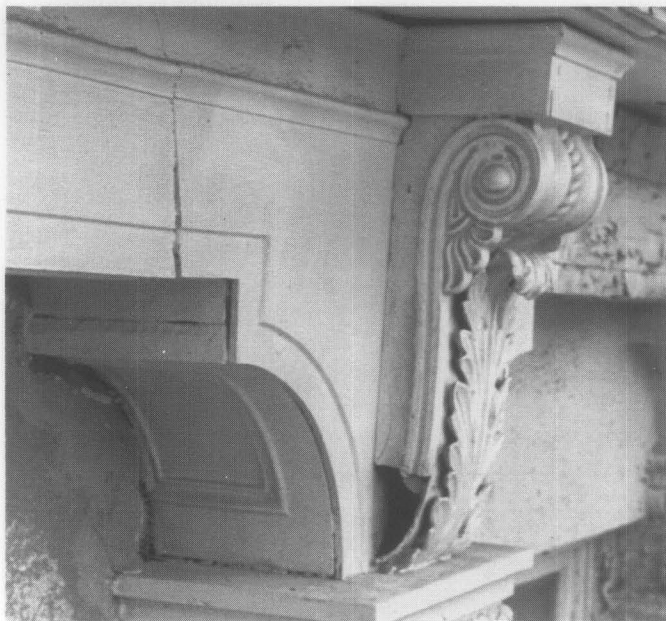
Fig. 8. Structural cracks, gaps at joints between components, and a large opening where part of the console bracket is missing are the problems evident in this cast-iron assembly. Photo: Ford, Powell & Carson.
