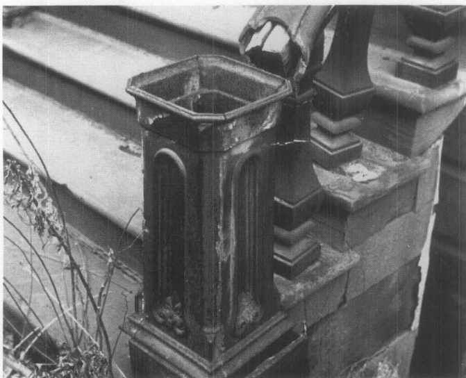
Fig. 15. In an effort to repair this stair railing, concrete was poured around the wood spacer inside the railing casting. Water penetrated the railing and reacted with the concrete to accelerate the corrosion of the iron. Photo: John G. Waite.
