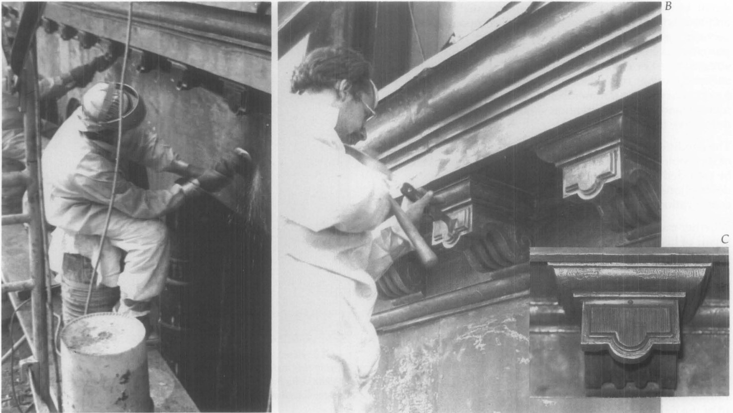
Fig. 13. Surface preparation may involve several different techniques. Where chemical paint stripping is involved, careful planning of the sequence of work and inspection by an architect or conservator to ensure strict compliance with the contract documents is important to minimize the risk of problems. After the chemical paste and paint was scraped off, the remaining paint and chemical residue were removed with a wire brush (a) and scrapers selected or cut to fit the shape of the iron surfaces (b). The surface was then wiped with solvent to create a completely clean surface prior to repainting (c). Photos: Raymond M. Pepi, Building Conservation Associates.
