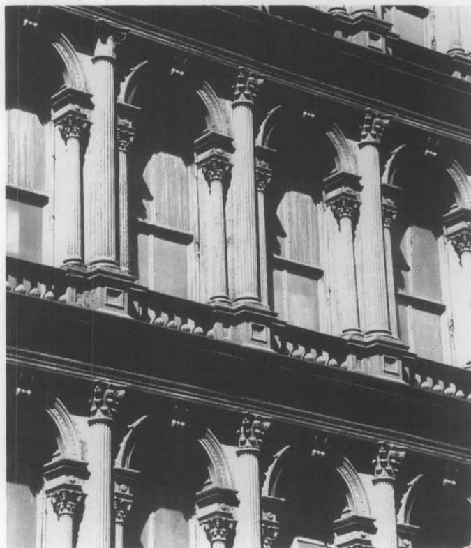
Fig. 1. The Haughwout Building in New York City is an excellent example of the quality and character of mass-produced cast-iron architecture. Once wood patterns were made, any number of elements could be cast, as was done with each of these repetitive bays. Photo: New York City Landmarks Preservation Commission.
