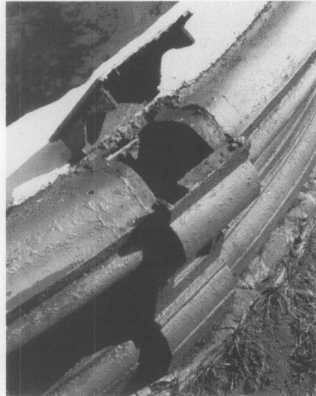
Fig. 9. Galvanic corrosion occurred where a patch of copper was installed alongside the cast-iron cap at the base of a fountain. The use of terne-coated stainless flashings with appropriate caulking would have been a more suitable repair. Photo: John G. Waite.
