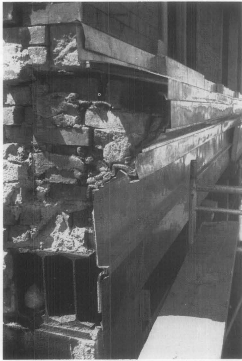
Fig. 18. This cast-iron storefront cornice was corroded beyond the point of repair, and could not be removed easily for replacement. Terne-coated stainless steel, the most durable metal for flashing cast iron, was applied to the cornice and fitted as closely as possible to the historic profile. Although painting is not necessary to protect terne-coated stainless steel, the cornice should be painted to be consistent with the historic character of the building. A primer which is compatible with the terne coating should be used. Photo: Dean Koga, Robert E. Meadows, P.C., Architects.
