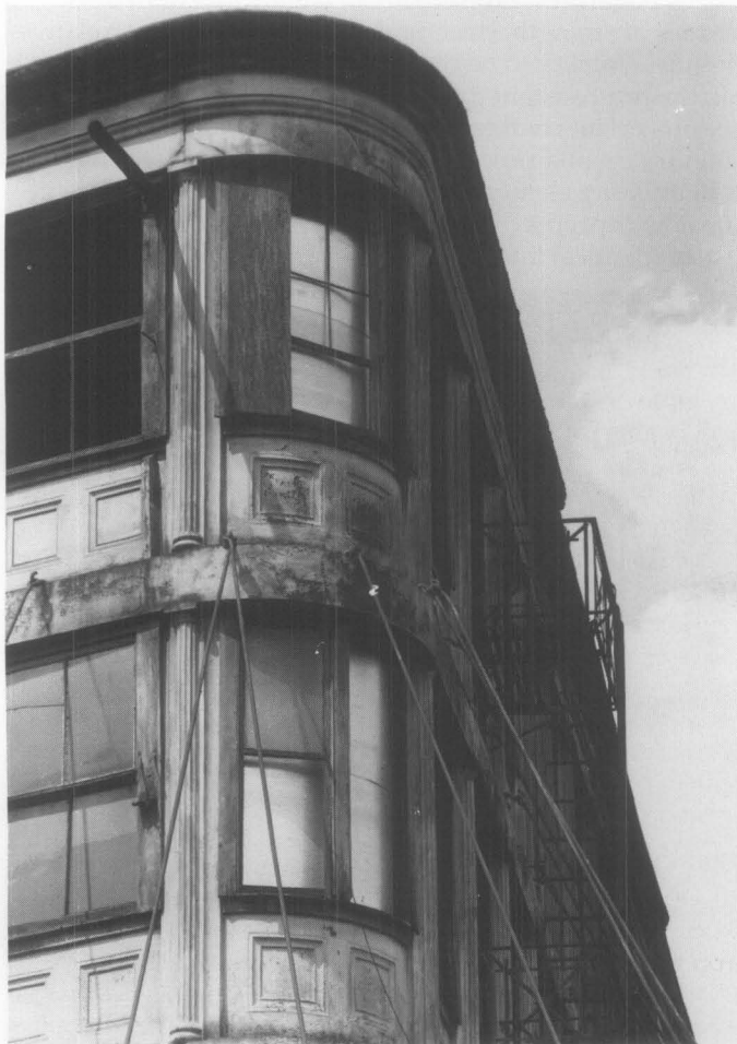
Fig. 2. The Edgar Laing Stores Block in New York City was designed by James Bogardus. It was the first building constructed with facades of self-supporting cast iron. This corner view shows the Doric-style engaged columns, panels, and spandrel beams; the loss of most of the original ornamental castings give it an austere look. As part of an urban renewal project, the facades were carefully disassembled in 1971 for later re-erection in another location—only to have its iron parts stolen for scrap. Photo: Jack E. Boucher, HABS Collection.
